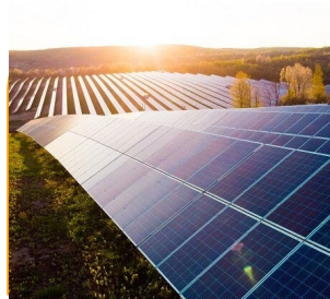
SOLAR PV PROJECT
