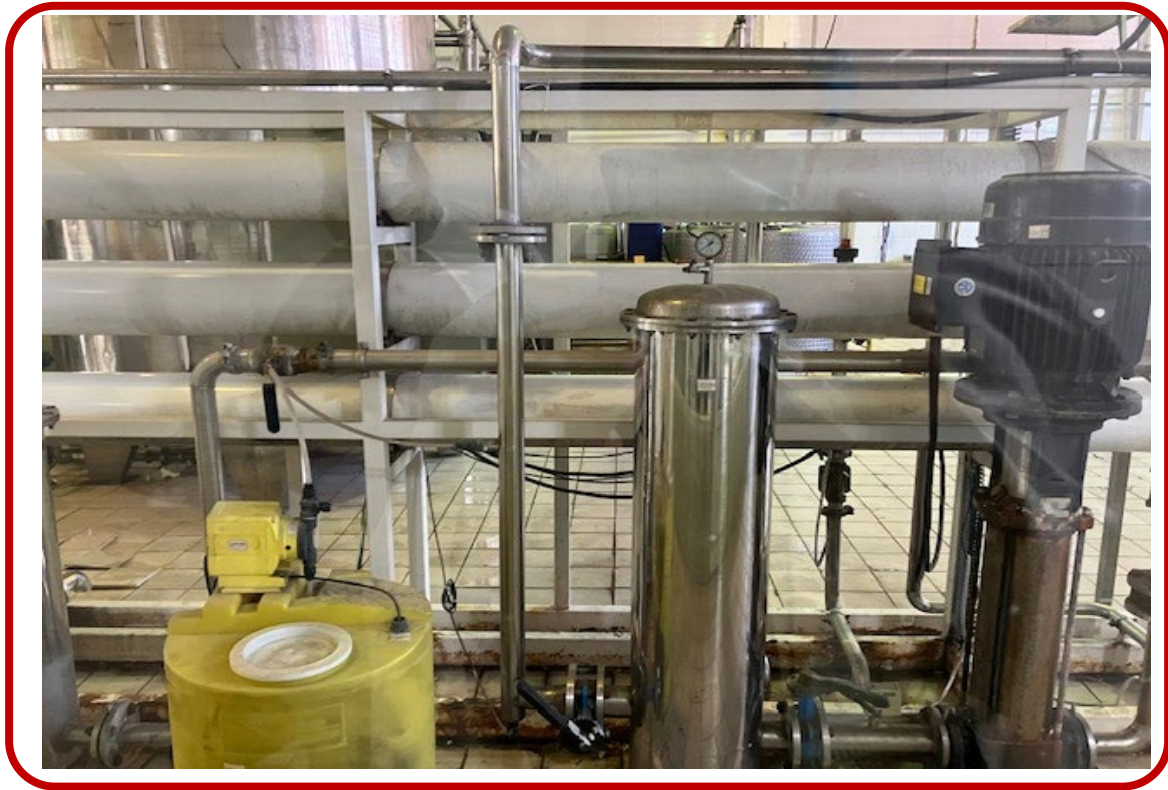
Process water treatment system made in China
