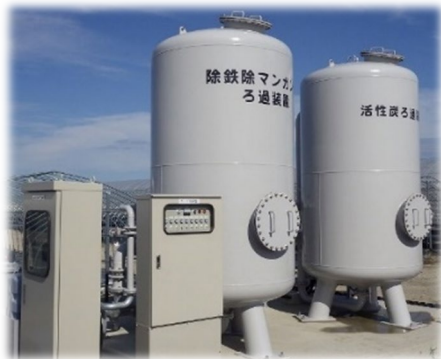
Sand filter & Activated carbon
