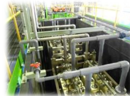
Submerged membrane filtration
