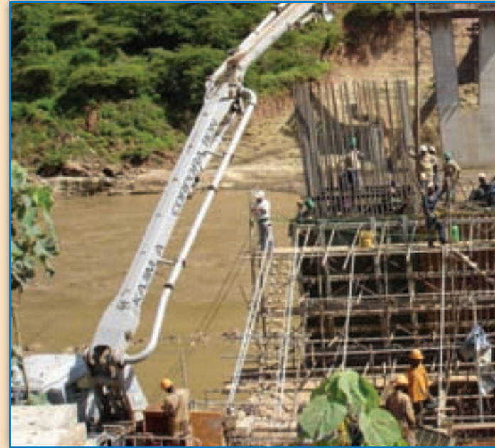
New Abay Bridge under construction in the Blue Nile Project. This is a Grant Aid project expedited by JICA
