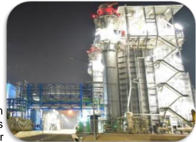
Central Termica de Maputo (CTM) constructed through this project
