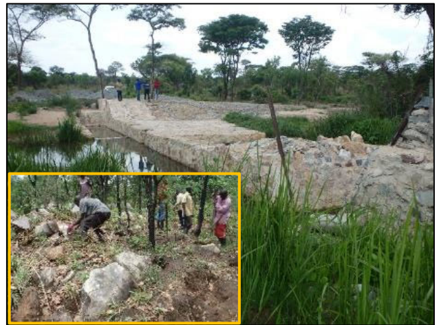
The remaining part is the right canal especially abutment and canal lining while the left canal is almost completed. The left down picture shows that farmers are collecting stones. (Mufulira district in Copperbelt province)
