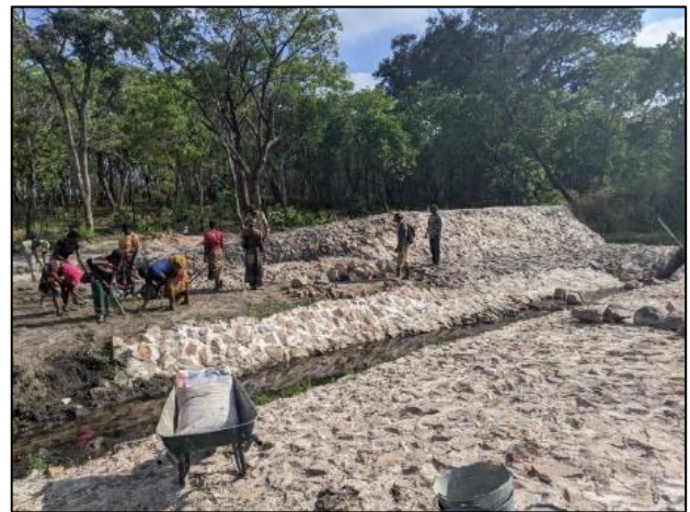
The picture shows that farmers are constructing slope protection of the right canal. They will conduct 20m additional lining for the right canal for the next year. (Kasempa district in Northwestern province)
