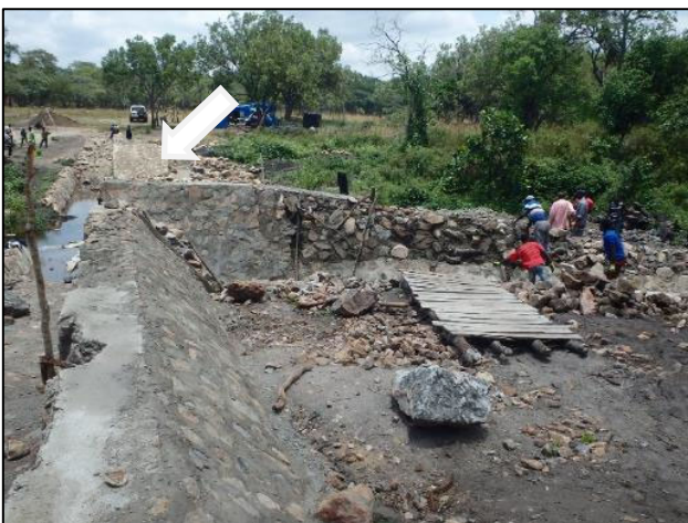
Construction of the right canal is almost completed. The remaining part is abutment of the left canal that the white arrow shows. The completion day will be around the beginning of December. (Mukushi district in Central province)
