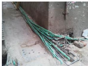
Spaghetti service pipes
