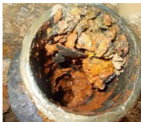
Internal Condition of Cut pipe
