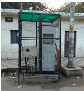
Local Measurement Stations
