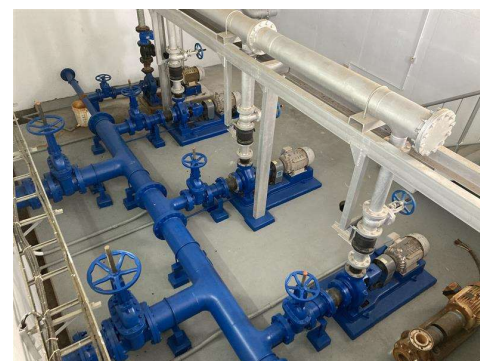
Well-maintained water treatment facility, a JICA’s Grant Aid for Water Supply in Corriverton, Guyana.
