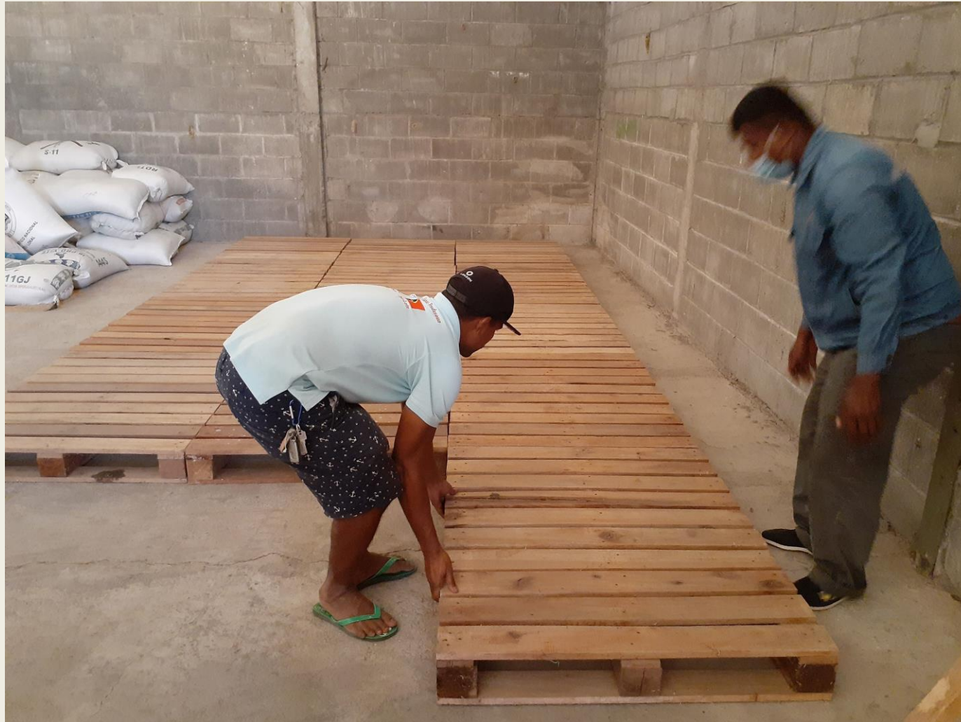
NLC Maliana Warehouse before rehabilitation
