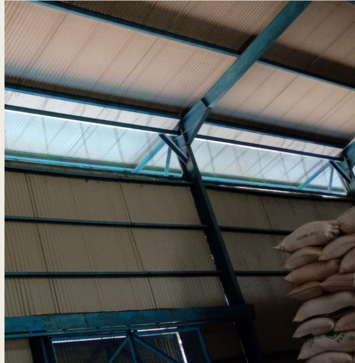
Bird prevention in Maliana Warehouse
