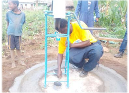
8. Putting the rope pump structure on the well cover and tightening bolts and nuts
