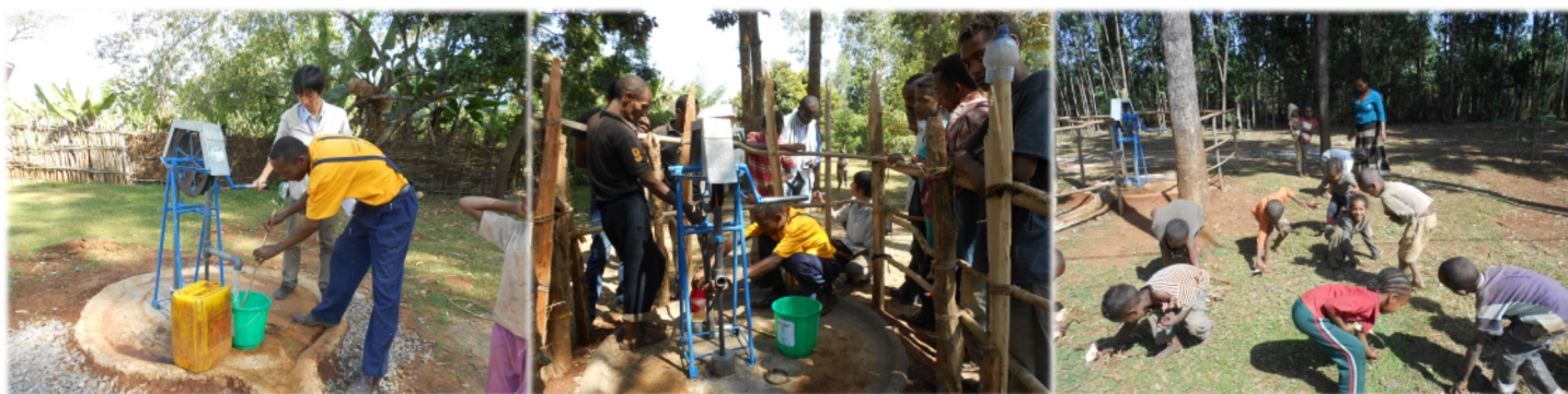
Zerihun (yellow Tshirt), from Dale Woreda Water Office, is mixing chlorine before putting to the well.
