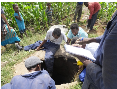
Measuring of depth and water level of well and checking well structure before installation of Rope Pump. 1
