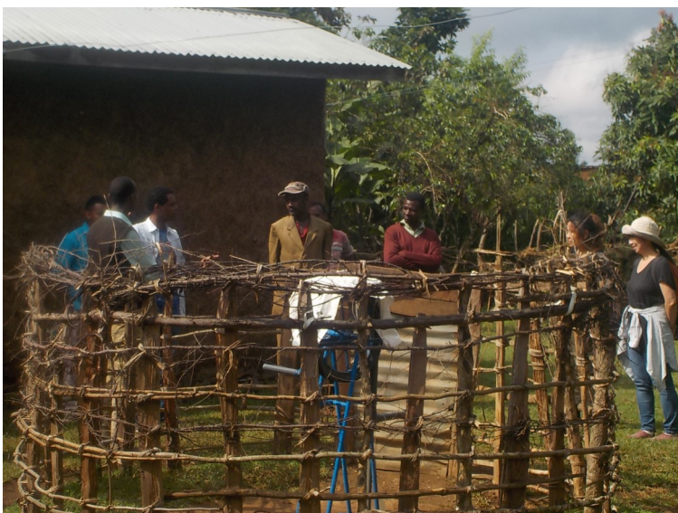
Ato Geremew, in center He made a wooden fence for protection the RP well by himself (Photo by WAS-RoPSS)
