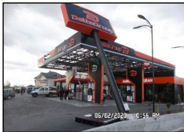
Signboard toppled by strong winds
