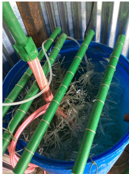
Figure 3.13. Actual image of how to set the Bio fringe in denitrification unit
