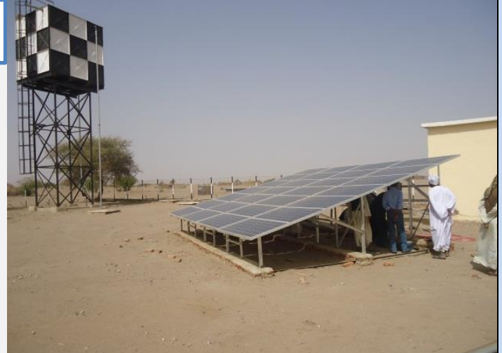
Solar panel in Banard village
