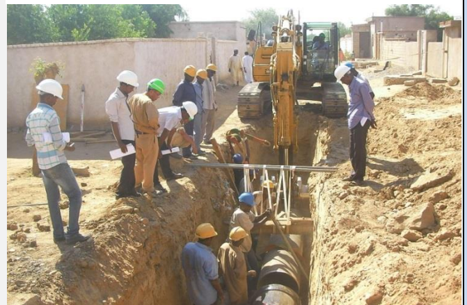
The SWC engineers are observing the laying transmission pipe of diameter 50cm and the distribution pipe of diameter 20cm.
