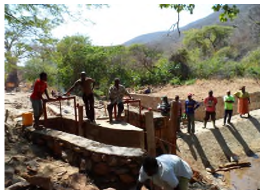
Mbeya Dissemination II : Iringa,D and PC Isaka is continuing Farmers' initiated Head work construction for 8 months.
