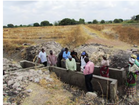
Training of Construction management for Misungwi district staff and Project Committee of Igongwa irrigation scheme.
