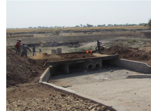
Rehabilitation work of Road crossing by ZITSU Tabora, Nzega district and farmers in Lusu irrigation scheme.
