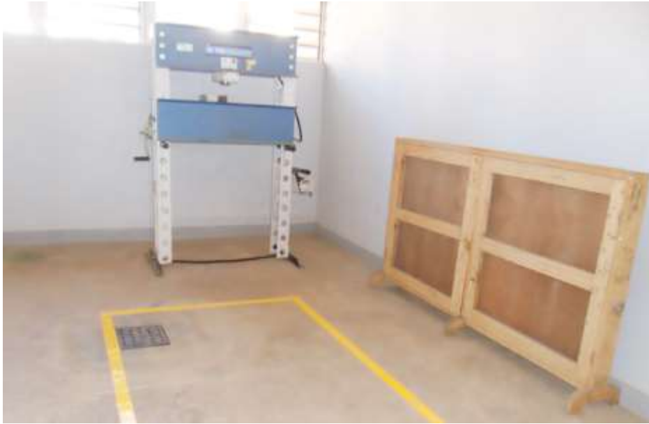
Testing machine room
