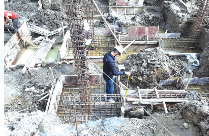
Supervision consultant conducting an interim inspection to verify the foundation as per approved design drawing.
