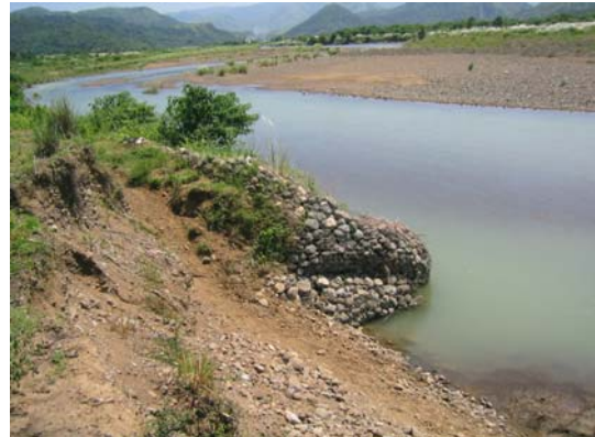
Figure 3 Damaged spur dike
