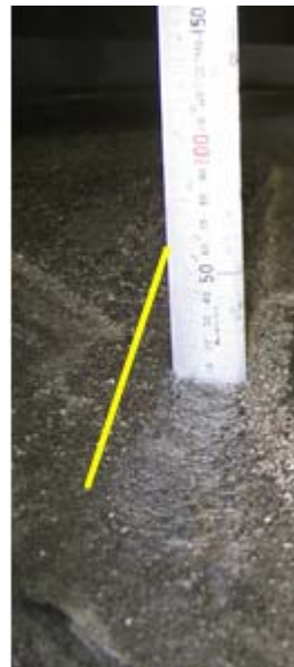
Figure 26, Depth of Scour
