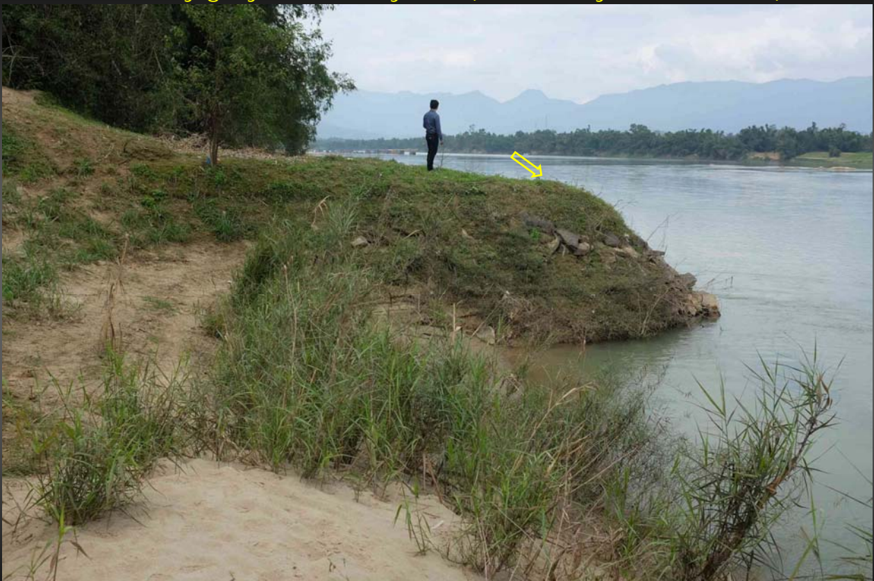
Masonry groyne after 4 years (Thanh Xuyen, 26/1/2014)
