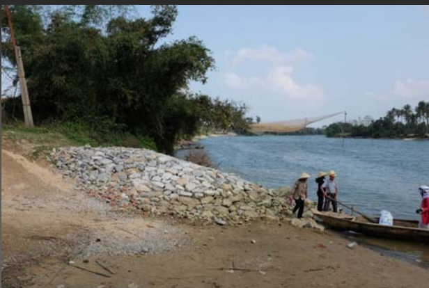
Continuous groynes at Quang Son commune on Rao Nan river, Quang Binh Province (29/1/2015)
