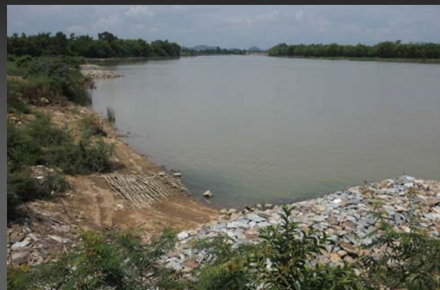
Combinational groynes at Duc La commune on La river, Ha Tinh province (14/7/2015)
