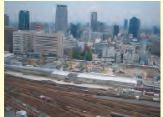
An urban renaissance project is underway on the northern side of JR Osaka Station. Many heavy machines are in operation.
