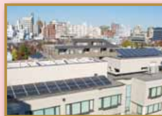
solar generating panels
