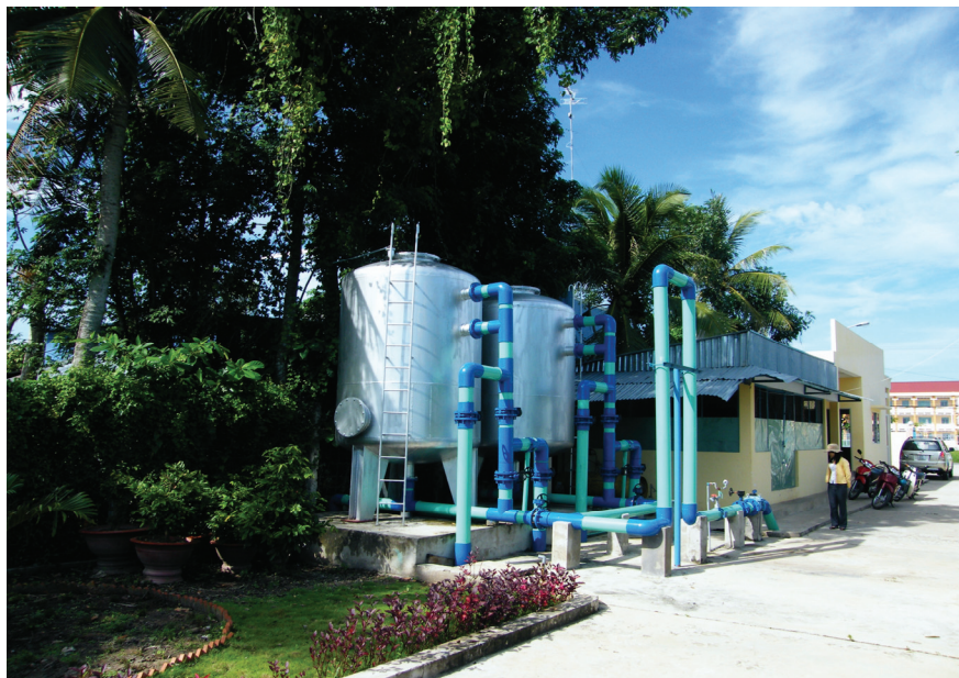
Water Supply Project in Phu Loc, Soc Trang province under SPL V.
