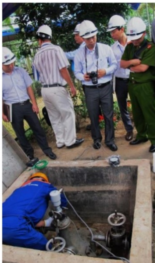
Demonstration of solution to avoid leakage of hazardous object
